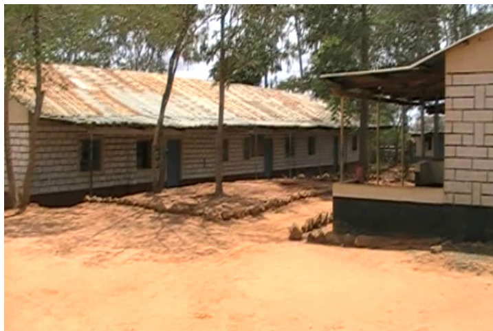
Two of the campus buildings requiring repairs. See details below.
